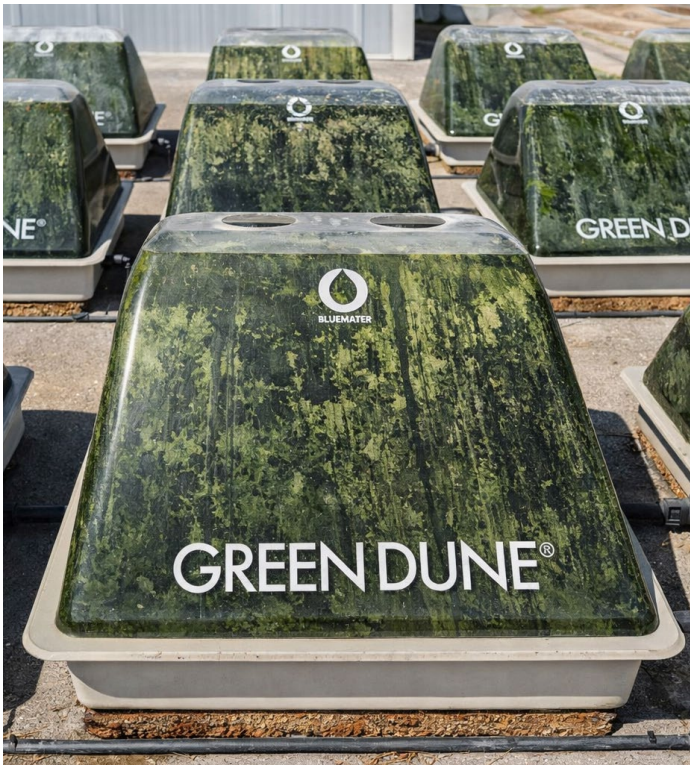
Figure 3: Photobioreactors GREEN DUNE® installed at the Thrasio Wastewater Treatment Plant, Greece.
