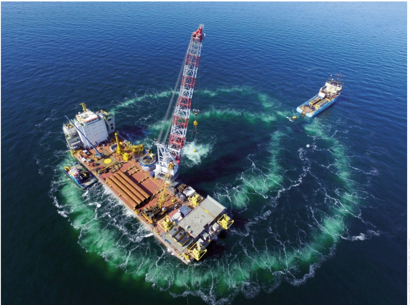
Double Big Bubble Curtain in action, used to mitigation sound propagation from pile-driving.
